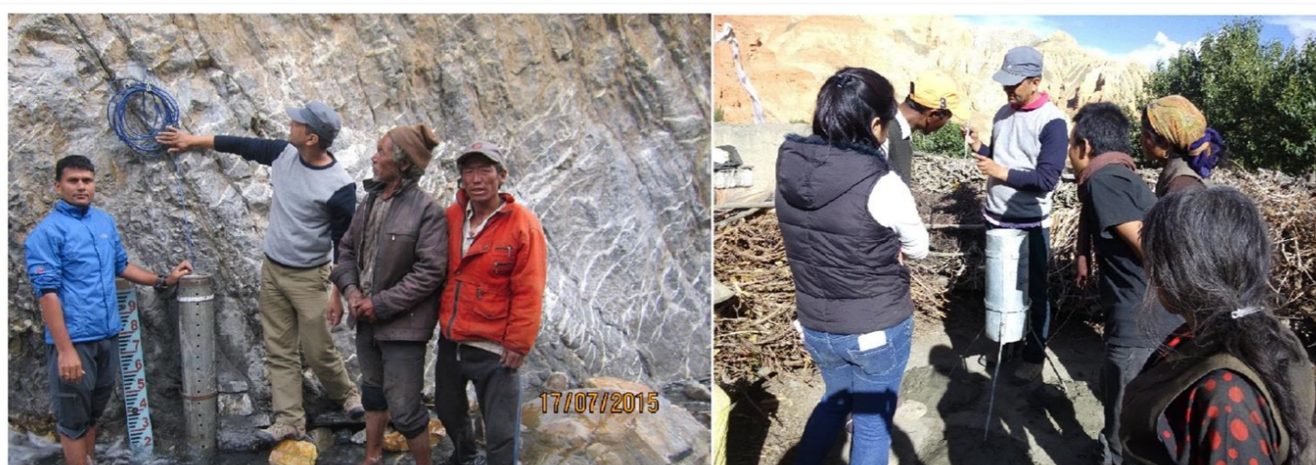
Figure 1. Installation of rainfall station and streamflow monitoring station at Lumbhuk stream, Nepal.
